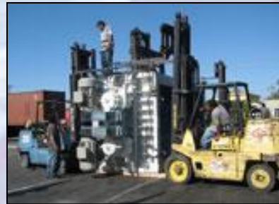
Power Plant - Kazakhstan
